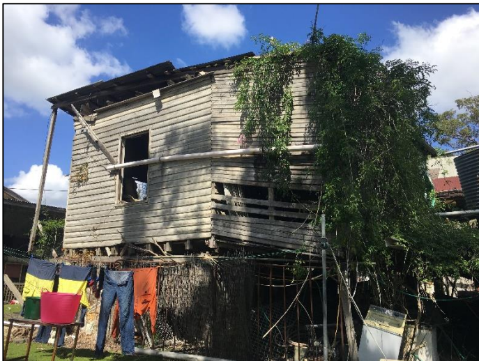
Plate 11: Dilapidated dwellings in the southeast portion of the site.
