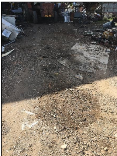
Plate 5: Oil staining within the large timber-frame shed
