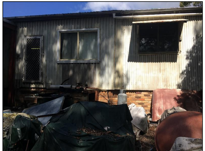
Plate 12: Dilapidated dwellings in the southeast portion of the site.
